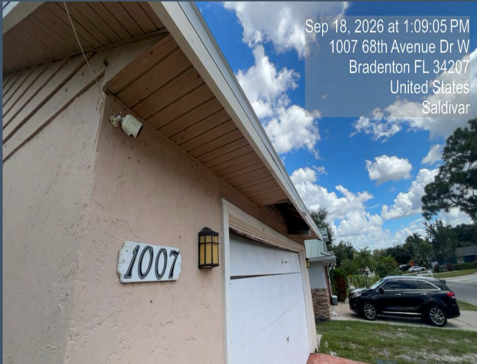
Picture depicts the missing soffit.
