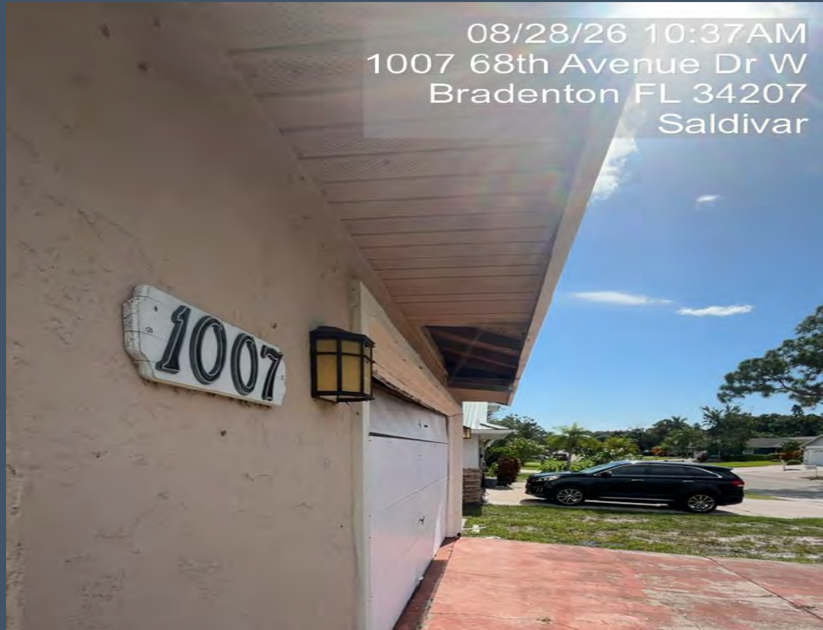
Picture depicts the missing soffit.
