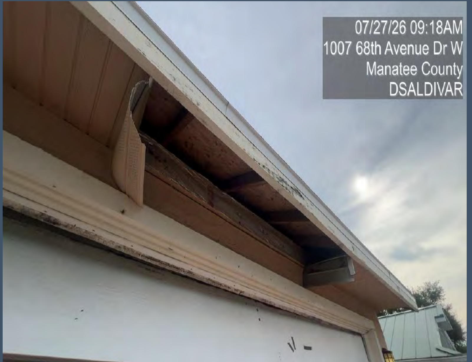
Picture depicts the missing soffit
